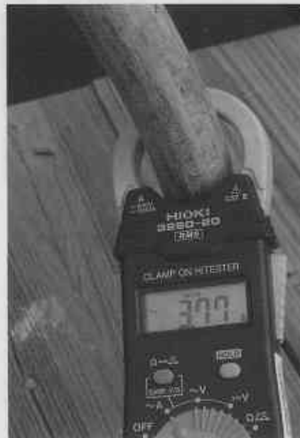
Marinas should install a ground fault detection system to prevent electrical ground fault accidents.
