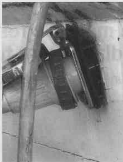
One thing all marina personnel can do to prevent marina electrical accidents is to visually inspect all electrical cords and outlets for any discrepancies listed in NFPA-303-2006.
